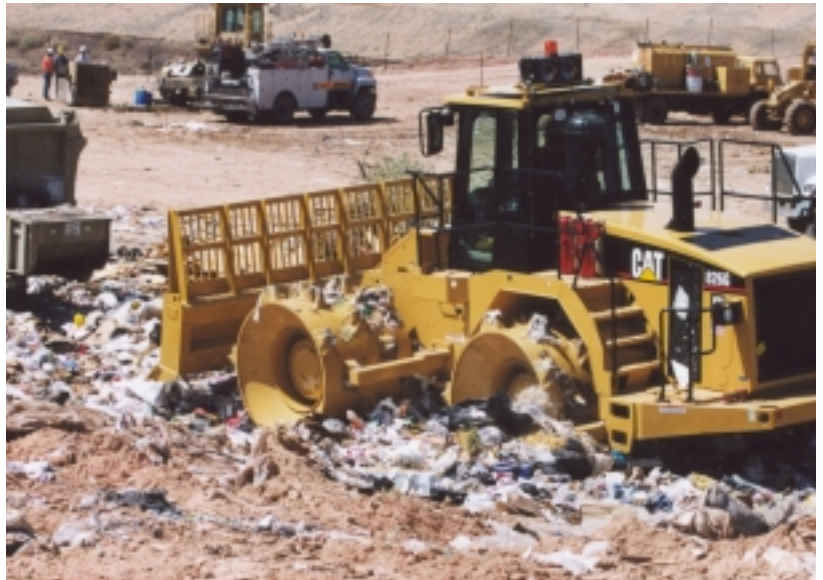
It didn't take long for the new 826G at Grey Wolf Landfill to get into the trash.
